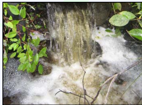
Example of an Impassable Perched Culvert in Ozaukee County
