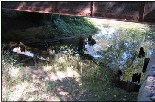
Sediment Deposited Below a Railroad Bridge
